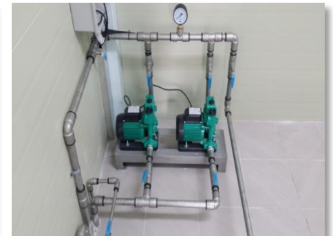
Sampling pump installation
