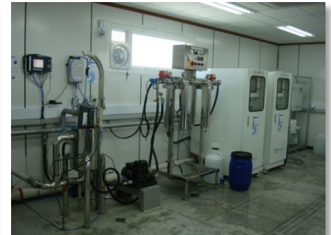
Measurement system installation
