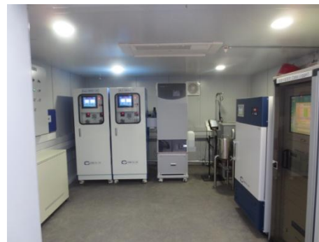
Measurement system installation
