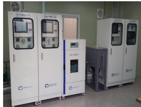
Measurement system installation
