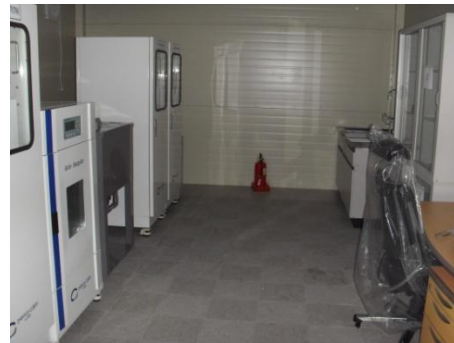
Measurement system installation
