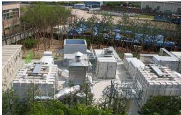
SH District Energy Site Sanggye area(2.8MW)
