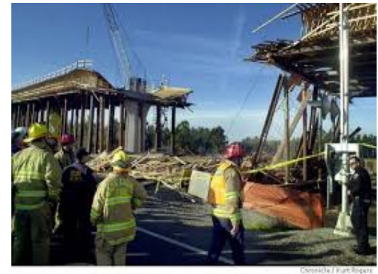
Collapse during Construction (2002) Casualty: 1, Injured: 7
